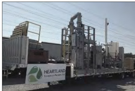
Electric Heater (pilot)
